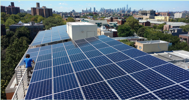
▲ Solar panels on a multifamily residential building. Bright Power, Inc. – U.S. Department of Energy.
